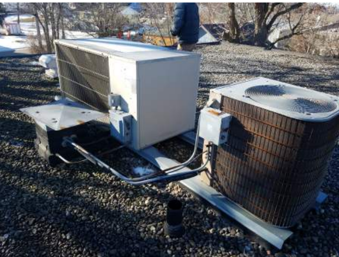
FIGURE 33: Rooftop and condensing unit appear to be about 20 years old, consider replacing in next 5 years.
