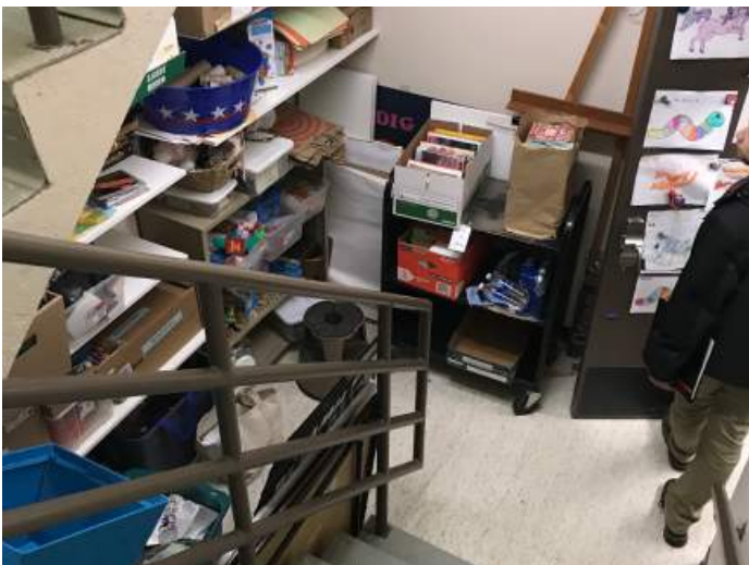
FIGURE 21: Per code, egress stairs should not be used for storage of any materials.
