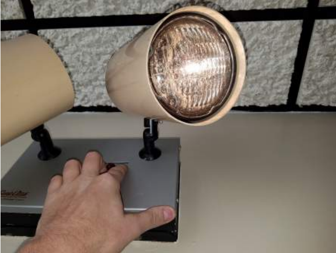
FIGURE 43: Emergency fixture, recommend replacement with leds.
