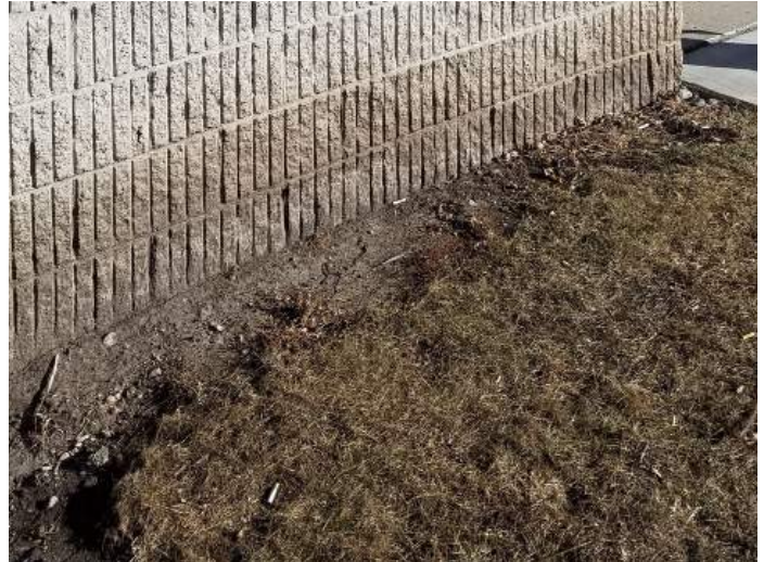
FIGURE 10: Evidence of water splashing/pooling along South face of building. Grading could be improved to minimize the standing water.
