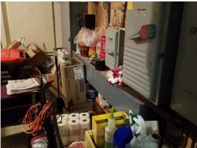
FIGURE 20: Items should not be stored within 3 feet of electrical panels and switched. Potential fire hazard.
