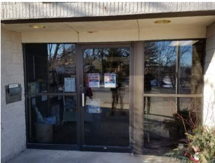
FIGURE 9: Aluminum windows and frames are in okay condition and appear to be original.
