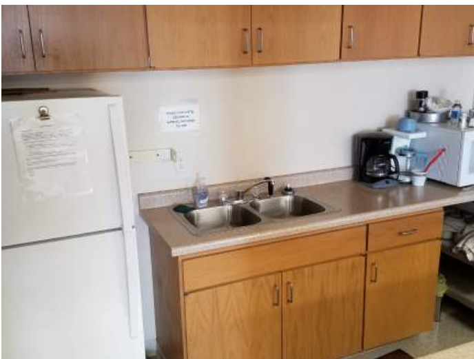
FIGURE 15: Accessible turning radius not provided in kitchenette area
