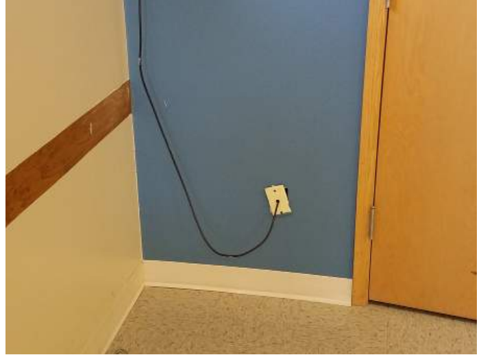
FIGURE 28: Cable receptacle is not securely installed in wall at Community Center.
