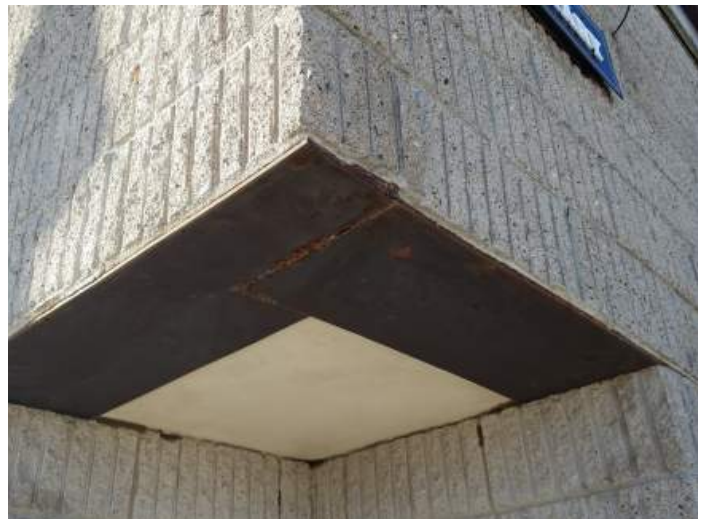
FIGURE 5: Steel lintel is rusting, structural integrity appears okay. Recommend repainting.
