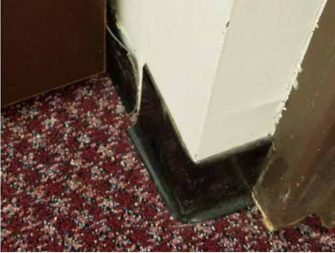
FIGURE 25: Vinyl base finish is separating from wall.
