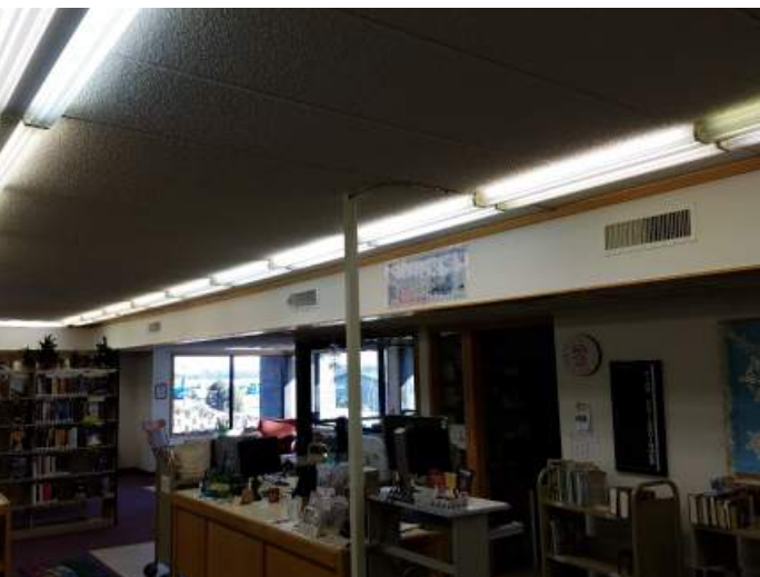
FIGURE 45: Existing ceiling mounted fluorescent fixtures, recommend led replacements
