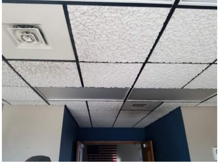
FIGURE 34: Supply ductwork is supplying air dirty enough to stain ceiling. Ductwork should be cleaned along with filter changes.
