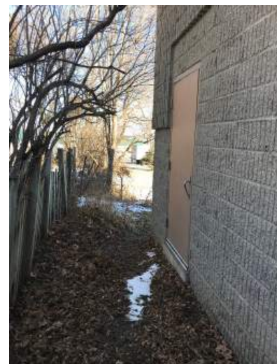
FIGURE 6: Exterior egress door from Community room does not provide an accessible means of egress, does not meet code requirements.
