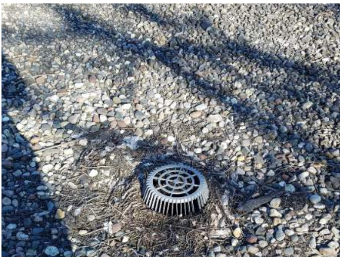
FIGURE 3: Roof drains are collecting debris and require cleaning. Recommend pruning adjacent trees to minimize debris accumulating on the roof.
