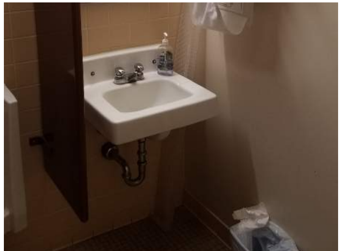
FIGURE 17: Men's restroom lavatory does not have pipe protection; toilet stall does not provide proper clearances for accessibility
