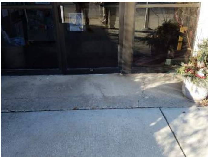
FIGURE 2: Concrete stoop at Library entrance is cracked and shifting.
