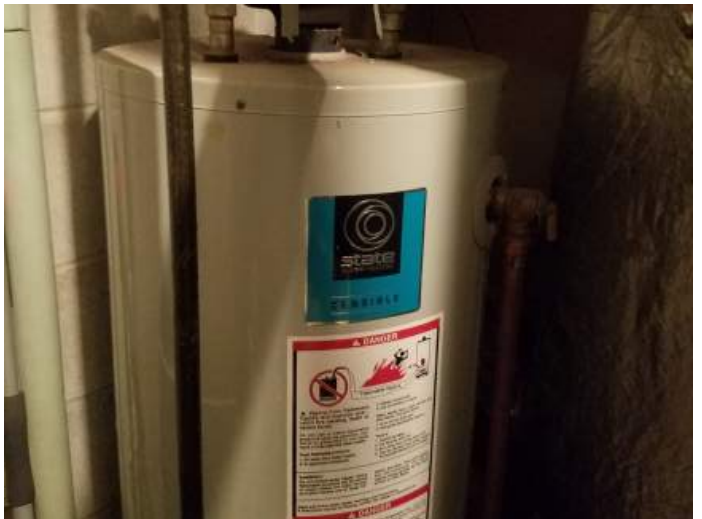
FIGURE 36: Water heater is in fair condition, but nearing the end of its useful life, consider replacing in the next 5 years.
