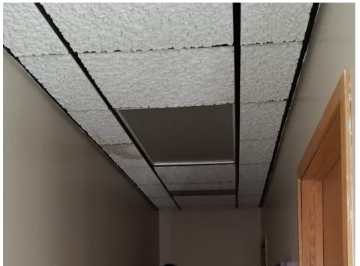
FIGURE 42: Fixture not functioning at time of assessment. Verify if working and replace if not.
