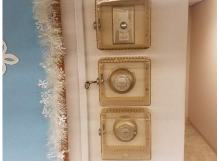
FIGURE 35: Non-programmable thermostats, recommend updating to programmable units.
