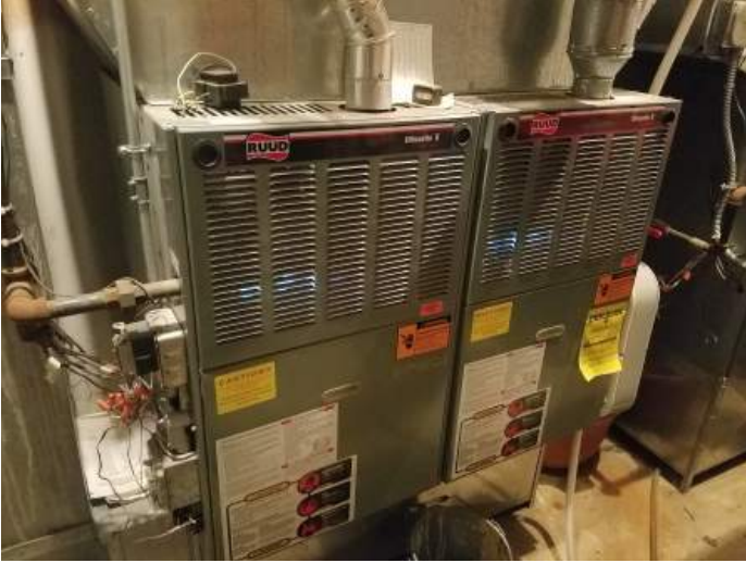
FIGURE 31: Furnaces are in good condition, near the middle of their useful life. Consider replacing these in the next 10 years.
