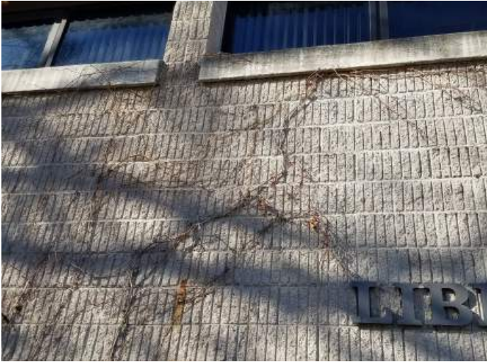
FIGURE 7: Vines have potential to damage masonry and should be removed from exterior surface of building.
