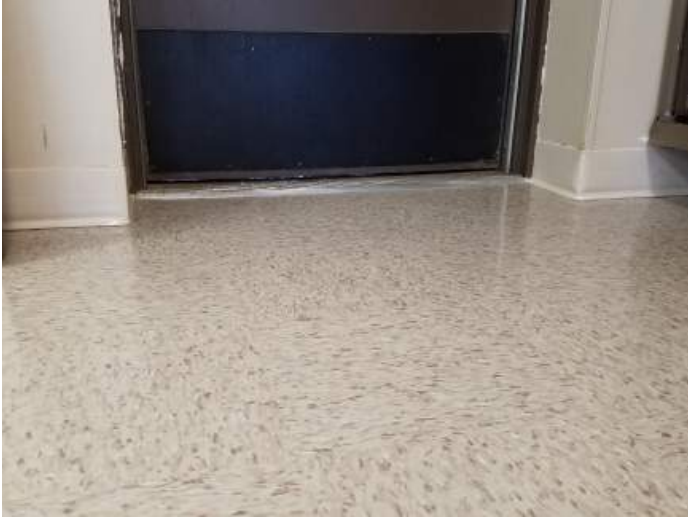
FIGURE 13: Exterior door at Community Room is missing weather stripping at threshold.
