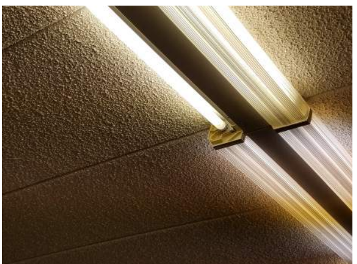
FIGURE 24: Missing bulb protection at ceiling fixture in Library. Current fluorescent fixtures are not ideal for reading and other stationary activities.
