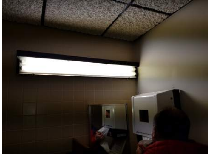
FIGURE 40: Missing light cover. Install cover to protect bulbs.
