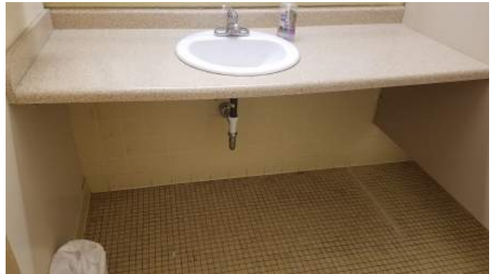
FIGURE 16: Women's restroom lavatory does not have pipe protection; toilet stall does not provide proper clearances for accessibility
