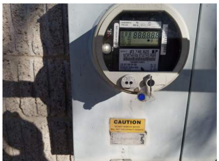
FIGURE 41: Utility meter, 200A service.
