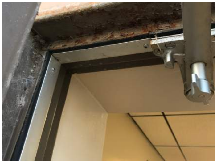
FIGURE 11: Corroding hollow metal frame at exterior door at Community Room; Frame should be repaired and painted.
