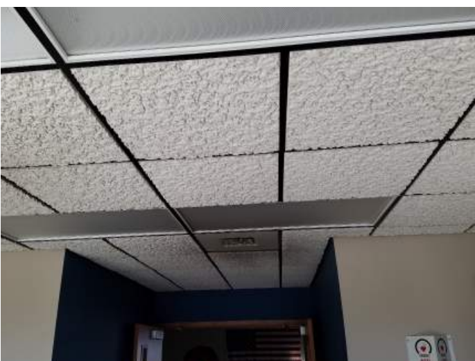
FIGURE 39: Fixtures not functioning at time of assessment. Verify if working and replace if not.
