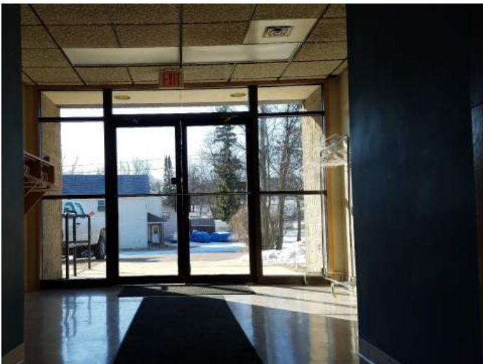
FIGURE 14: Aluminum entry doors are missing weather seals.
