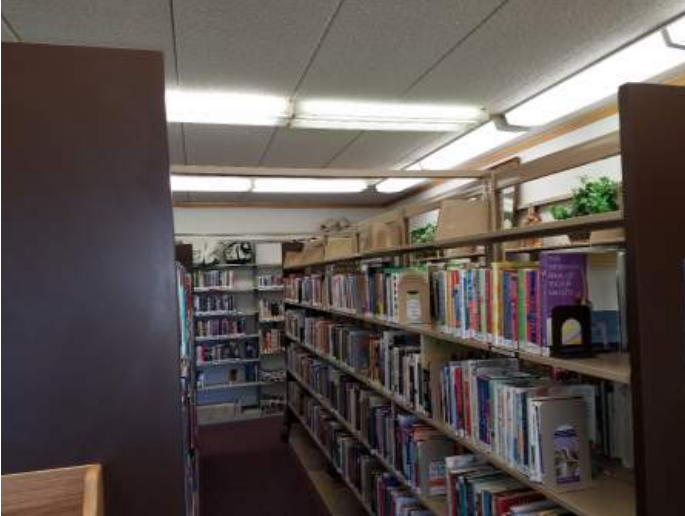
FIGURE 37: Emergency fixture needs to be relocated for better coverage and visibility.
