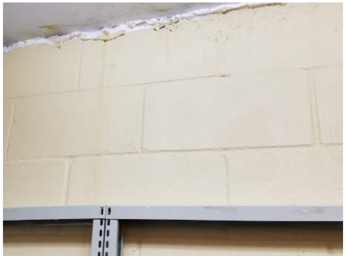
FIGURE 23: Evidence of water intrusion at South wall of Library space.
