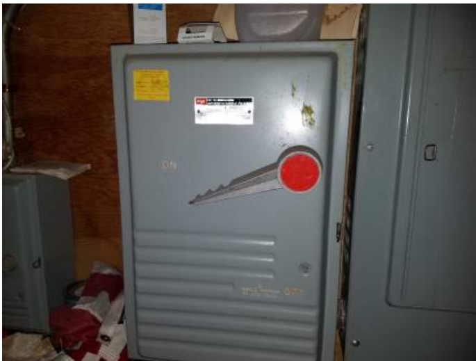
FIGURE 38: Power panel and disconnect. Life expectancy 30yrs.
