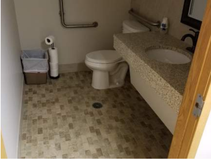
FIGURE 19: Library restrooms are not accessible, do not provide clearance for turning radius and clearance at door.
