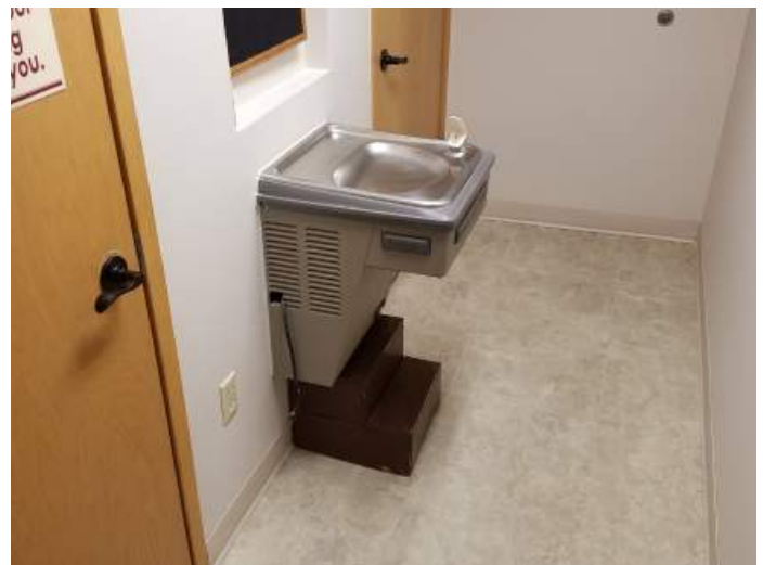
FIGURE 18: Hallway to restrooms does not provide proper clearances to access restrooms with protruding drinking fountain and current door swing
