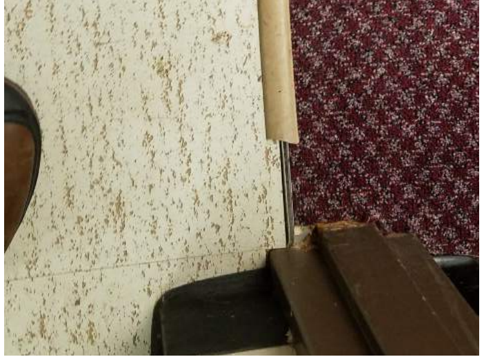
FIGURE 22: Flooring transition strips cracked and missing.
