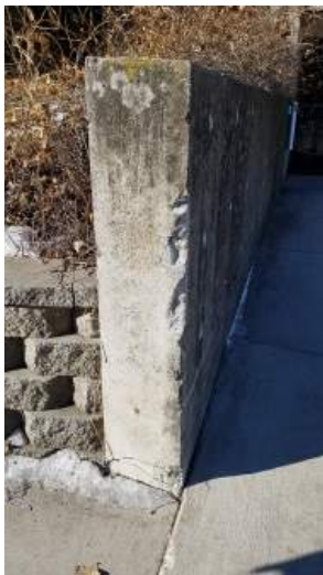
FIGURE 8: Damaged concrete retaining wall.
