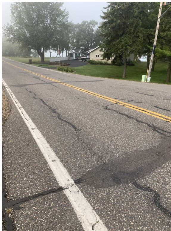
Figure 5: CSAH 7 Existing Road Condition
