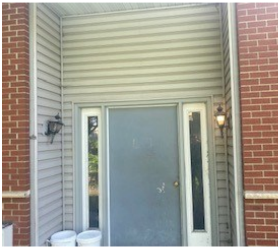
Broken entry light
