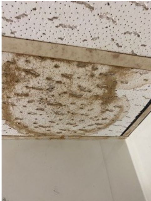
Water/mold damage in bathroom
