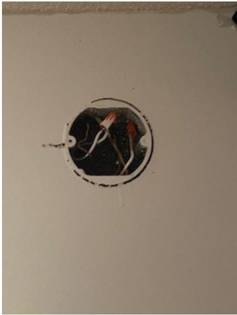
Exposed junction box
