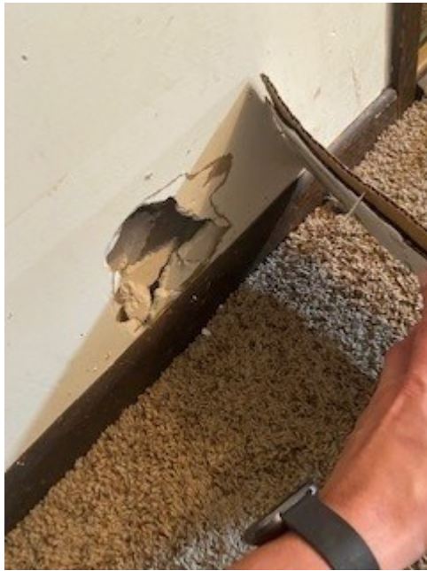
Hole in sheetrock
