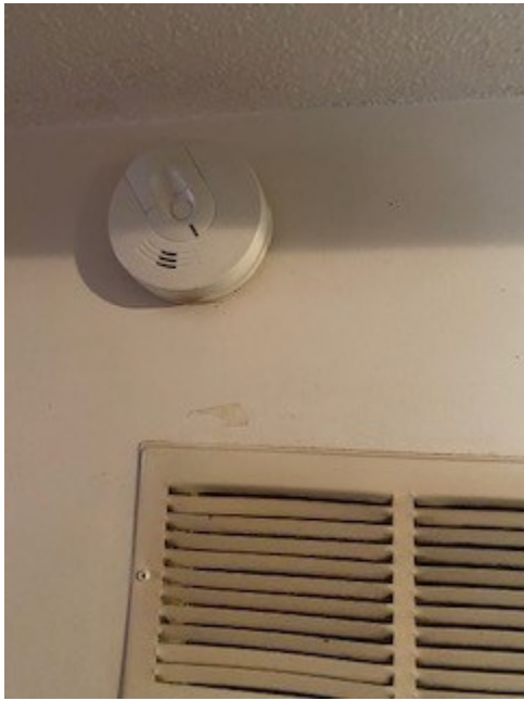
Inoperable smoke detector
